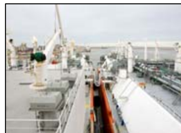
Figure 1: High pressure gas comes ashore via a jetty-mounted articulated gas loading arm. Photo courtesy of Exceleerate Enerav.
